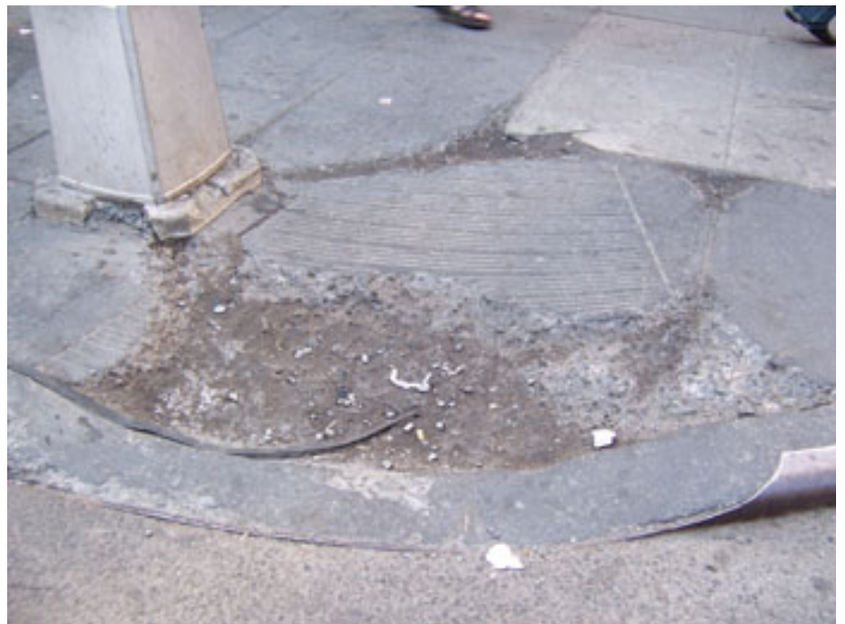
Eroded curb cut Photo by Jean Ryan
