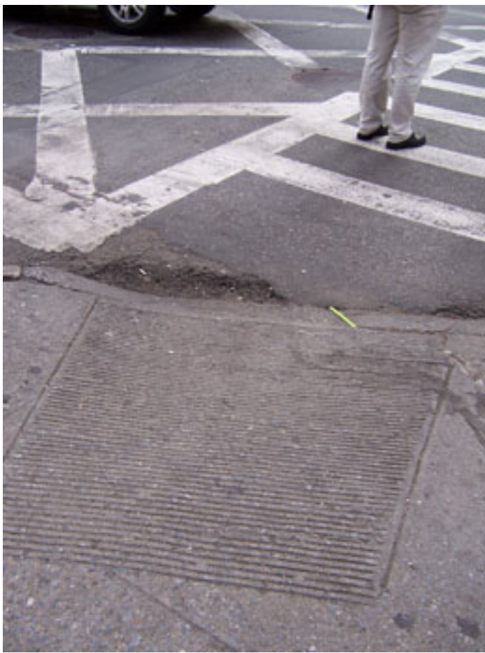
Hole at foot of curb cut Photo by Jean Ryan
